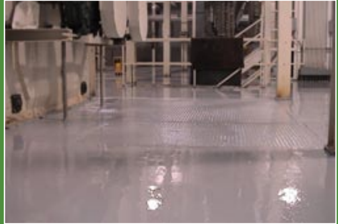
Feed Mill Floor
